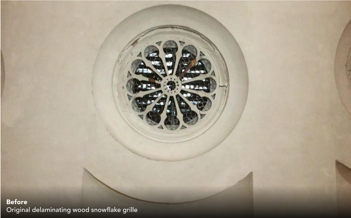
Before Deteriorated and missing original snowflake grilles
